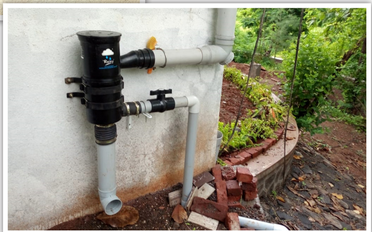
Rainwater Harvesting Unit at Bungalow (Pashan Area)
